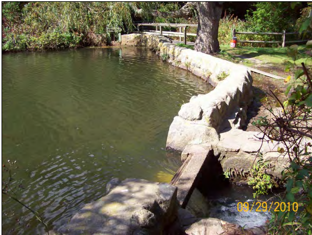
Photo No. 1 – Upstream stone masonry wall with spillway in foreground, viewed from right abutment
