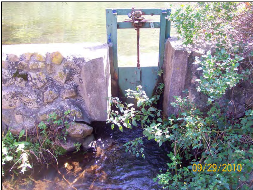
Photo No. 5 – Low level outlet slide gate
