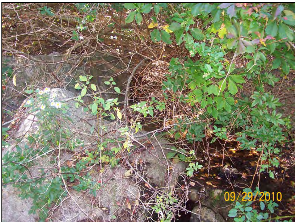
Photo No. 6 – Left abutment area with leakage visible on right
